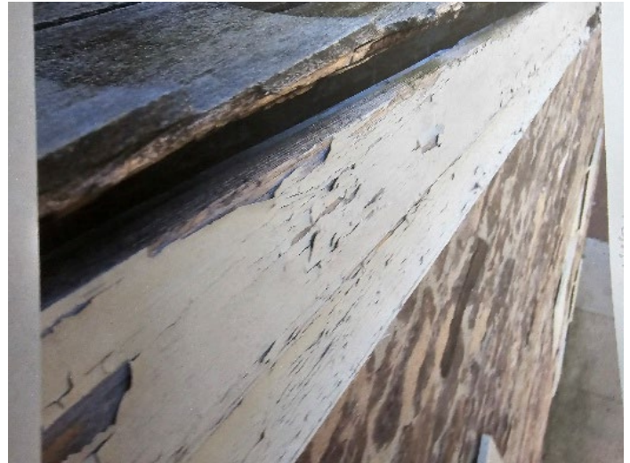
The Court Inn Roof Damage
